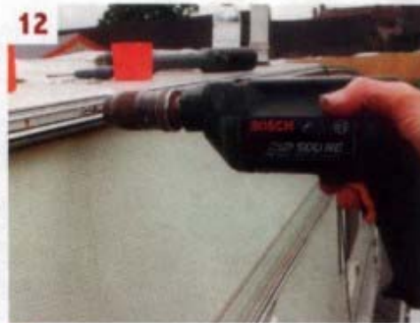
12 ■ The channel was temporarily re-fixed so that fresh holes could be drilled to receive replacement screws
