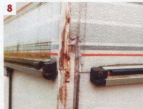
8 ■ Several sections underneath the rail looked pretty susceptible to weather penetration
