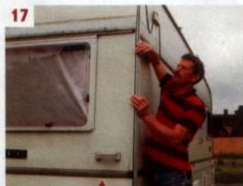
17 ■ Each section was pressed firmly into the bedding sealant, taking care to ensure there was continuity in the channelling groove
