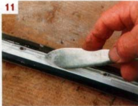
11 ■ An old fish knife is my favourite tool for getting into tight spaces such as removing sealant from the rear side of the channelling
