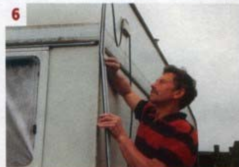
6 ■ A lower section was removed first and it was noted that some remnants were still in fairly good condition
