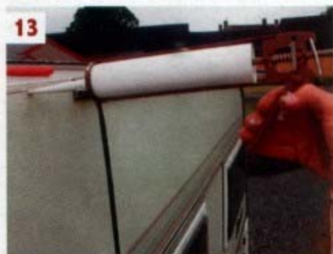
13 ■ Sealant was pumped into all the holes, both the original ones and the new holes for replacement fixings
