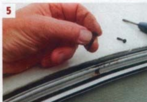
5 ■ A few rusting screws had lost their threads as well – a sure sign that water is starting to creep in where it's not wanted
