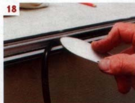
18 ■ The plastic trim was re-inserted next. Then a thin bead of Sikaflex 221 was injected along the roof edge of the awning rail itself
