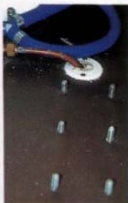
2 6mm dia holes were drilled down through the floor and the coachbolts pushed up through the underfloor plate.
