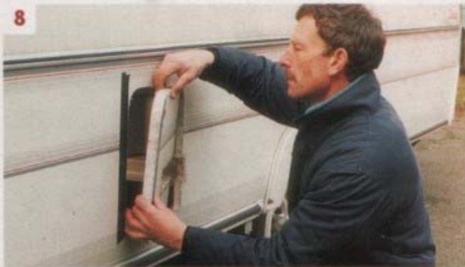
8. The section of sidewall removed needs to be kept safe for later installation within the frame of the cassette toilet access door
