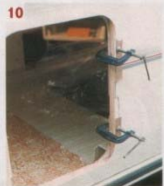
10. A wooden frame fits inside the void and is bonded in place
