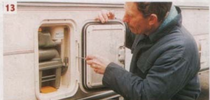
13. Make sure the hinge side of the door is nearest to the front of your caravan. Screw the toilet door in place on its bedding of sealant
