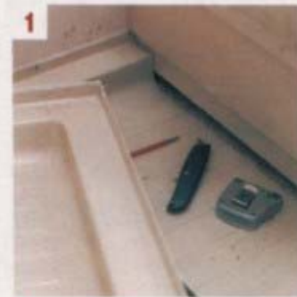
1. Reducing the shower tray in size to make space for the toilet
