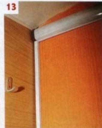
13 Inside the toilet I ran the cables in miniature ducting and secured it to the partition with self-adhesive backing
