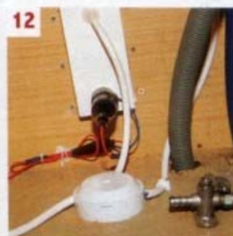
12 The mains cables were secured with cable clips and the 12V cables with cable ties
