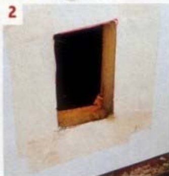
2 I used my powerfile to open the hole to size. Note the use of rockwool insulation
