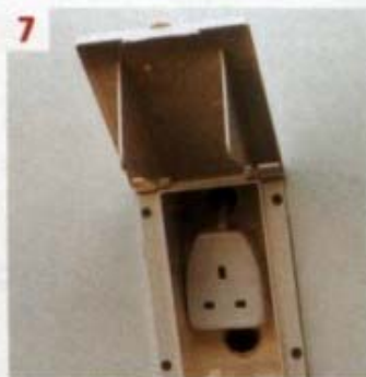
7 The cable was pushed through into the van and the socket secured to the rear of the housing
