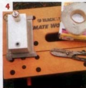
4 Mastic sealing strip was applied to the rear of the housing flange and I used bradawl to pierce holes
