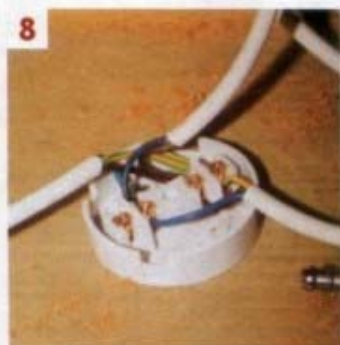
8 Inside the van I cut the existing supply cable and then reconnected it together with the new cable
