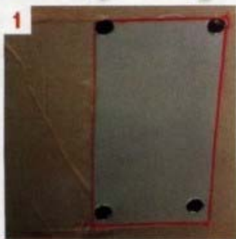
1 I marked the cutting line and masked the area before drilling a 10mm dia. hole at each corner
