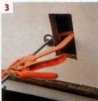
3 I used 25mm square timber to provide a firm base for the socket housing and clamped it in place
