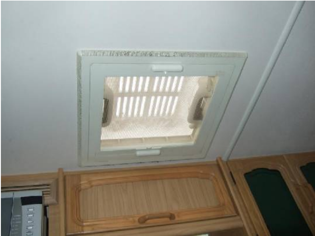
This was the old and black spotted roof vent
