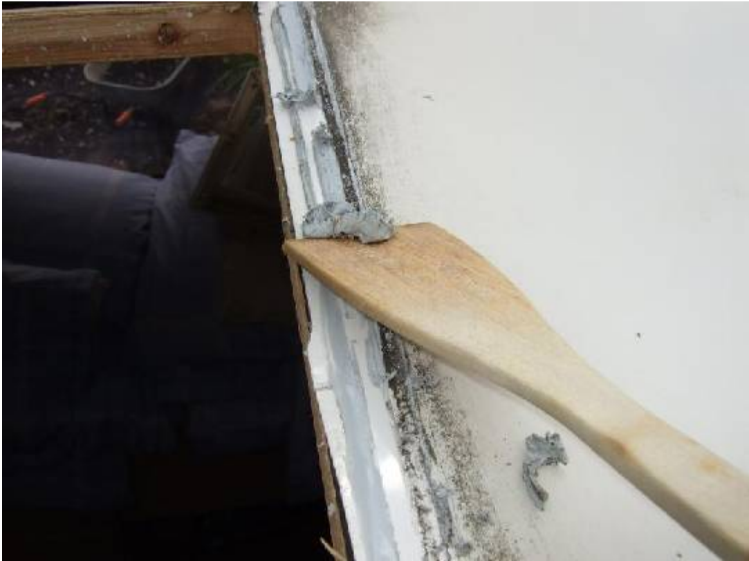
This will leave a lot of the old mastic that needs scraping off. An old wooden spatula will help!
