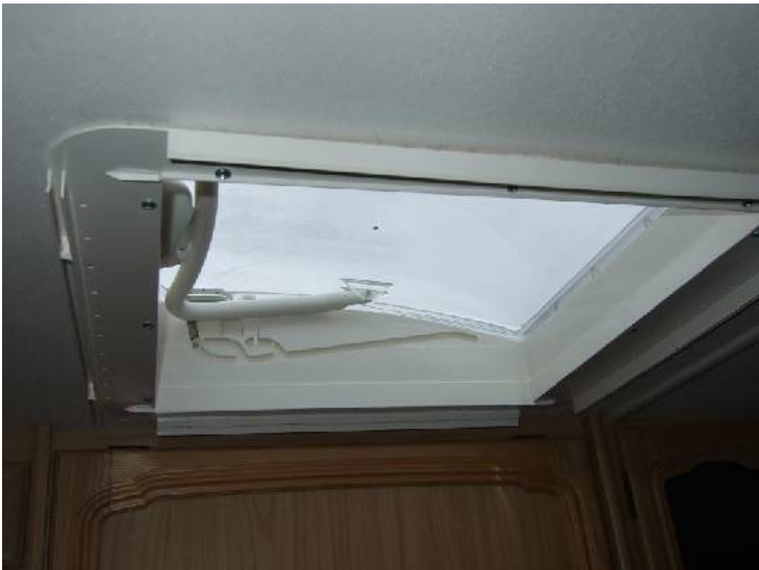
Next two pictures show the inner surround fixed to the top vent. I had to cut 4mm of each lug before fitting.
