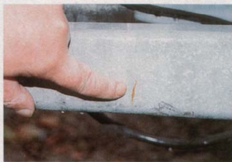
Deal with rust before winter really bites. Prepare affected areas well before applying a good-quality, zinc-based paint
