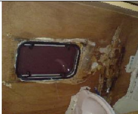
The extent of the damp in the bathroom
