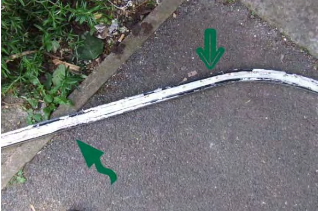
indicating the start of the water ingress.
