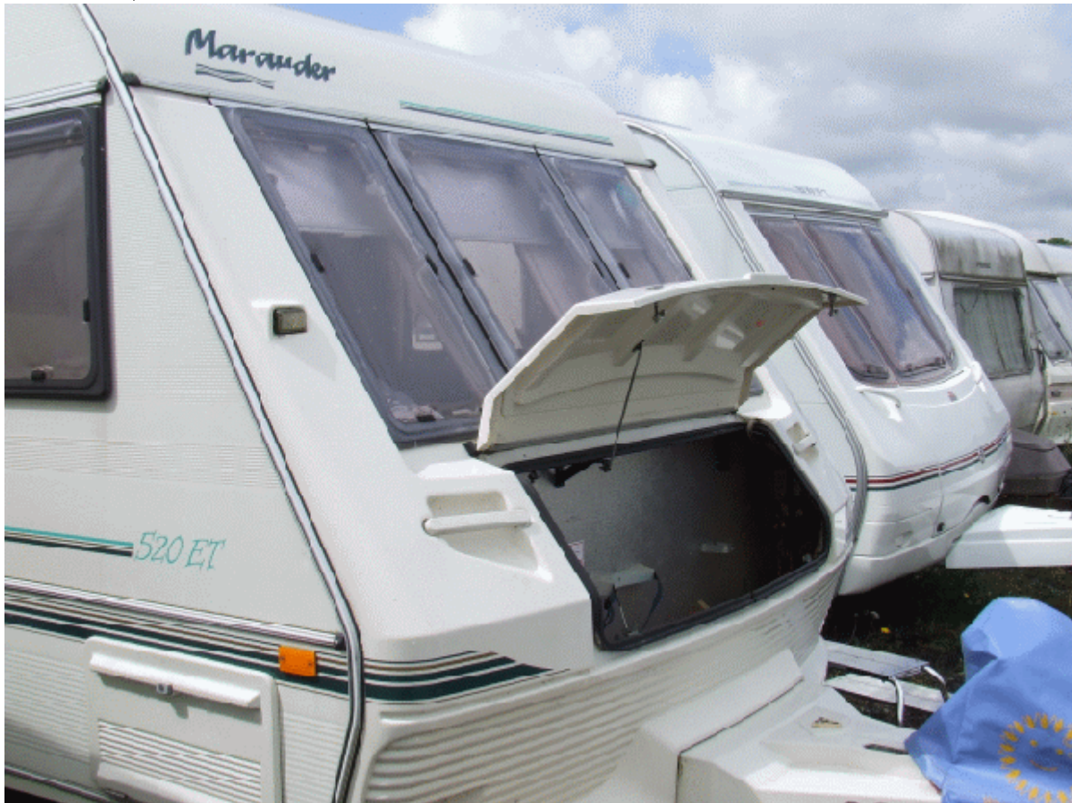
The naughty spot was in the lower corner of the bulkhead compartment. In the shadow.
