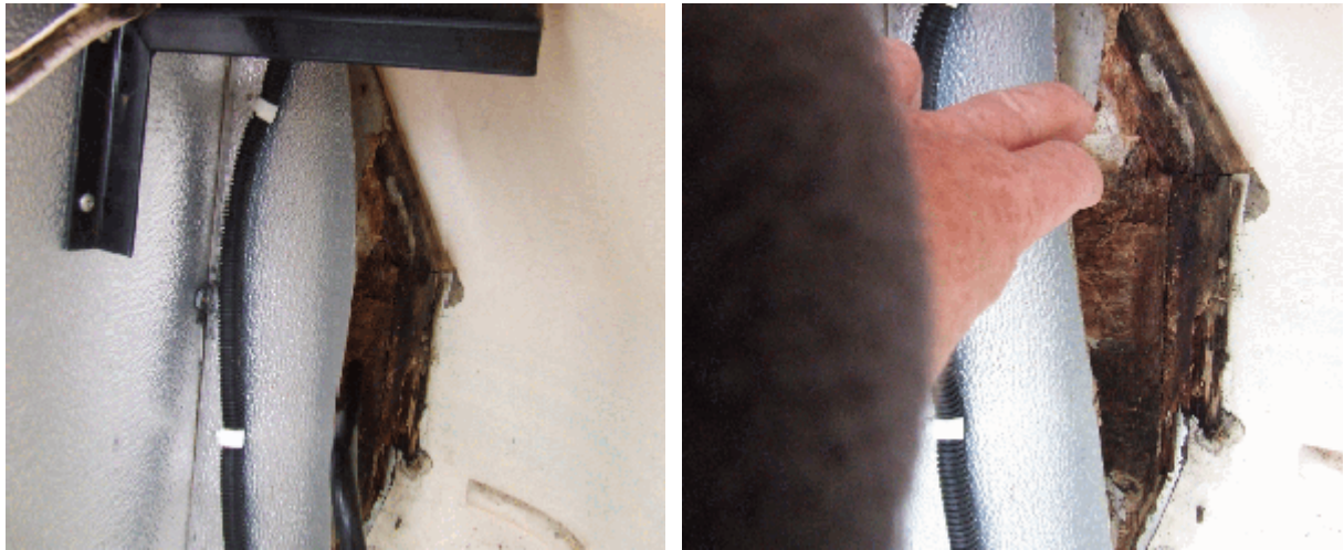
The sheet peeled back reveals the rotting and sodden timber in the nearside bulkhead,
